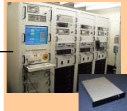
Controller and power supplies
